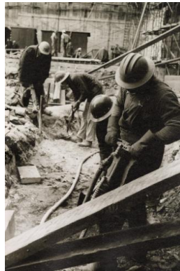
Title: Constructing workers jack-hammering and digging Date: c. 1955 Primary Maker: Jacques Lowe Medium: Vintage gelatin silver print
