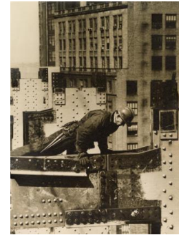
Title: Construction worker climbing over metal beam Date: 1955 Primary Maker: Jacques Lowe Medium: Vintage gelatin silver print
